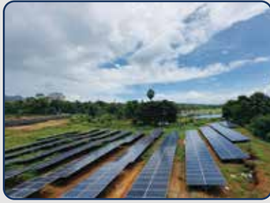
1.5MWp Solar Power plant at Nenmara Palakkad
