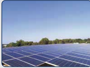
2MWp Autokast Limited Cherthala
