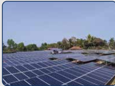
400kWp Solar power plant at Manjeshwaram
