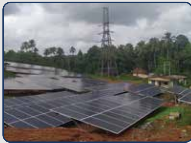
400kWp Solar Power Plant at Cherpulassery
