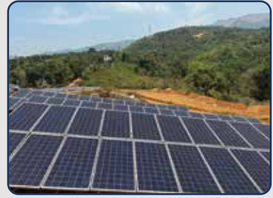
2MWp Solar Power Plant at Mananthavady
